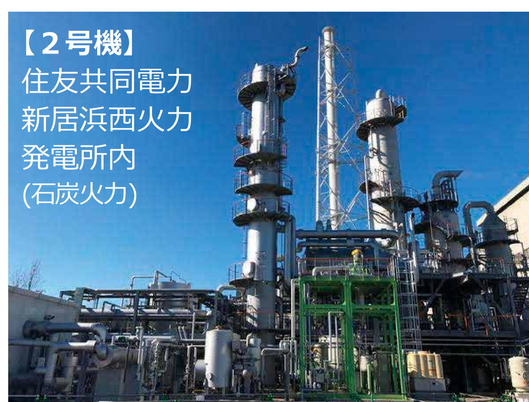
【2号機】住友共同電力新居浜西火力発電所内(石炭火力) https://www.eng.nipponsteel.com/business/environment_and_energy_solution/escap/escap/
